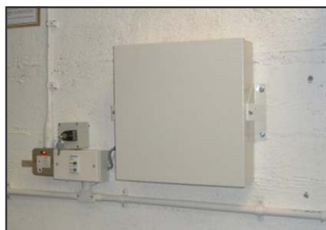
Battery Back Up System
